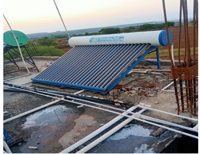
d) Solar Plant
